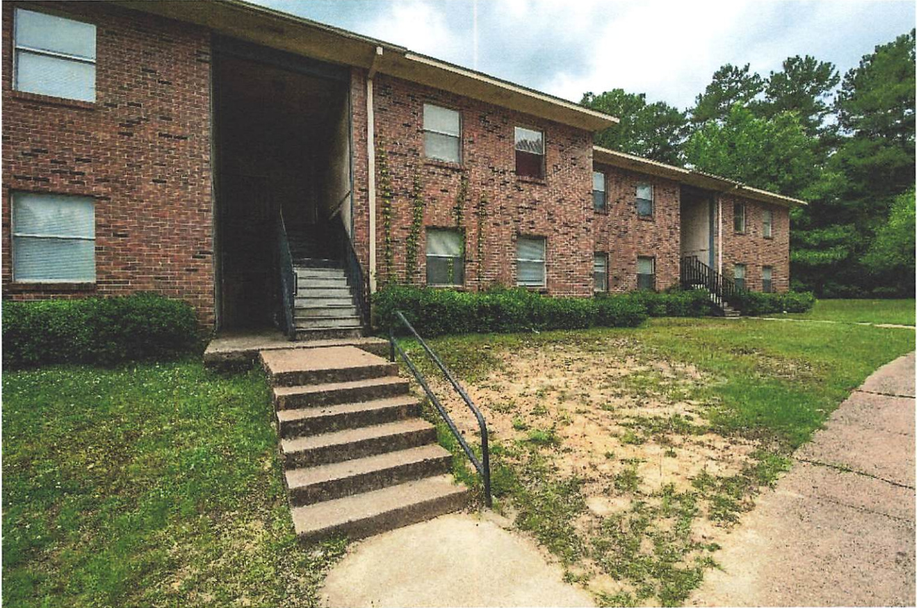
Entrance steps with inadequate handrails and side protection
