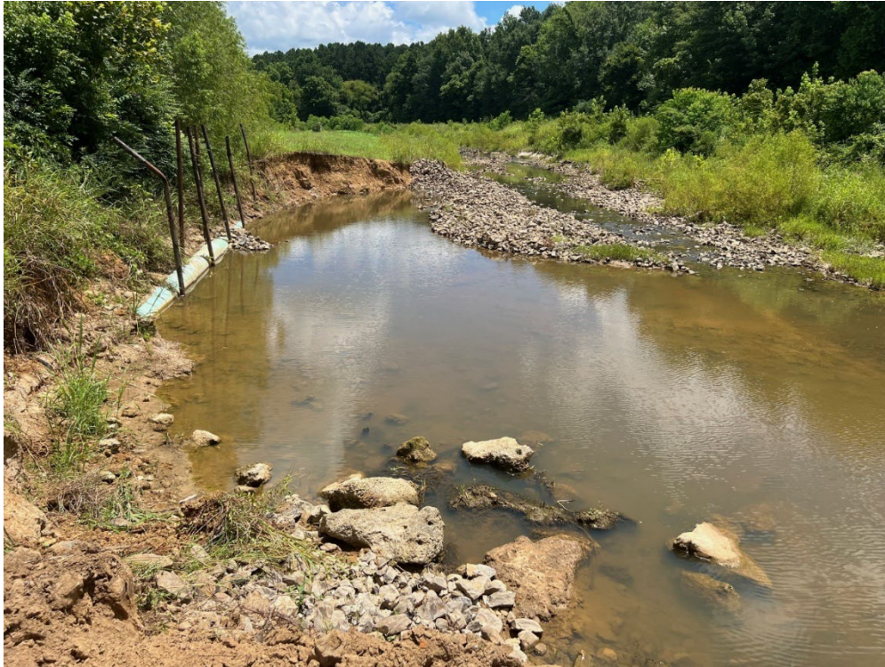
Head Cutting Along Streambank; Additional Sewer Line Exposed Since Preliminary Survey
