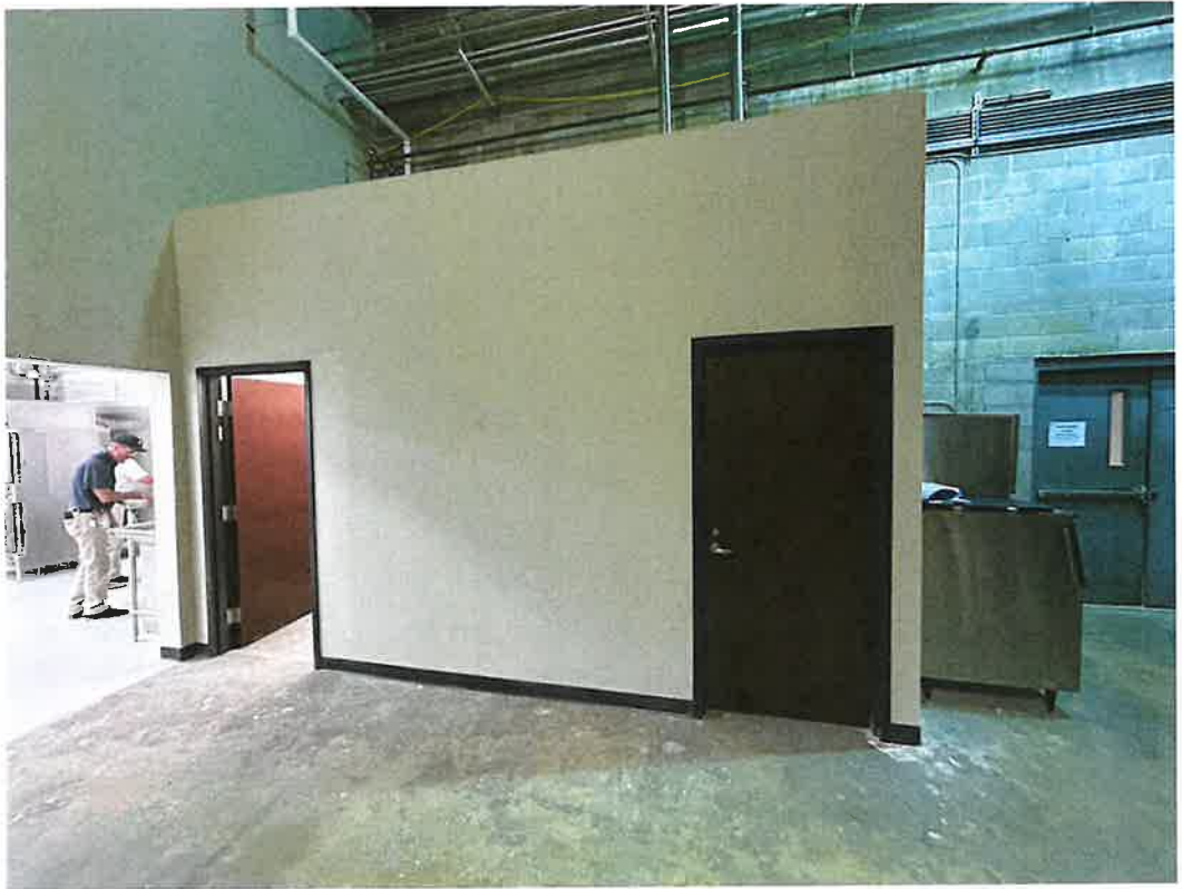
No Ladder/Paint Touch Up
